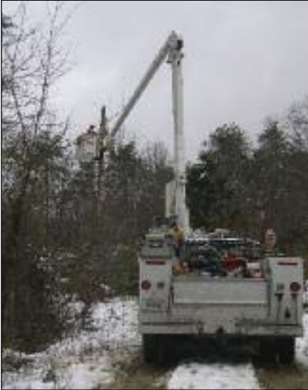
A crew braves uncomfortable conditions to further the restoration effort. When crews arrived at outage locations, they were often forced to maneuver the bucket trucks into position amid slick snow and slimy mud.
