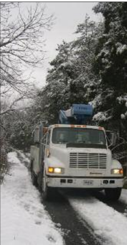
After the snowfall, Holston EC trucks are among the first vehicles to cross the county roads. Cutting fallen trees out of the roadway was often necessary to get to the downed power lines.
